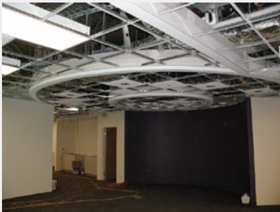
Devecka Construction was chosen to build this unusual round-wall design for ITXC
